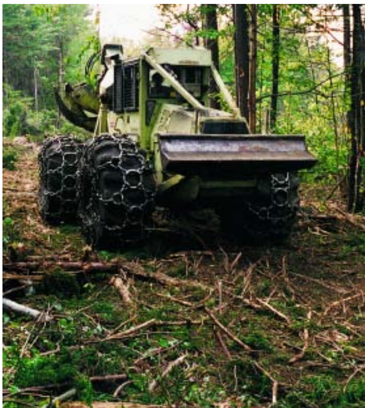
Brush on skid trails, as well as frozen ground, helps minimize soil disturbance and rutting.
